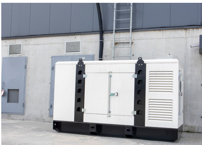
Coupling fitted between the engine and alternator.
